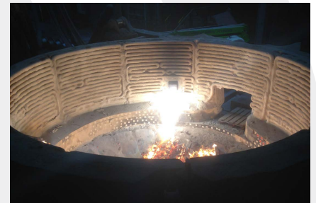
Furnace view with VLB in operation – burner mode with flat angle ...
