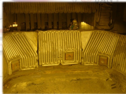
VLBs with copper case integrated in shaft furnace side wall
